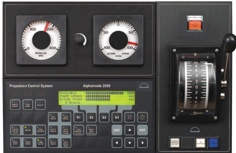
Fig. 9: Bridge manoeuvre panel – main bridge
